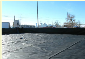
Tank Pad Lining
